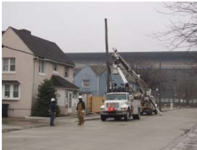
Line crews remove the last of the old above ground telephone lines before taking down the wooden poles that lined Spruce Avenue for at least 5 decades.
