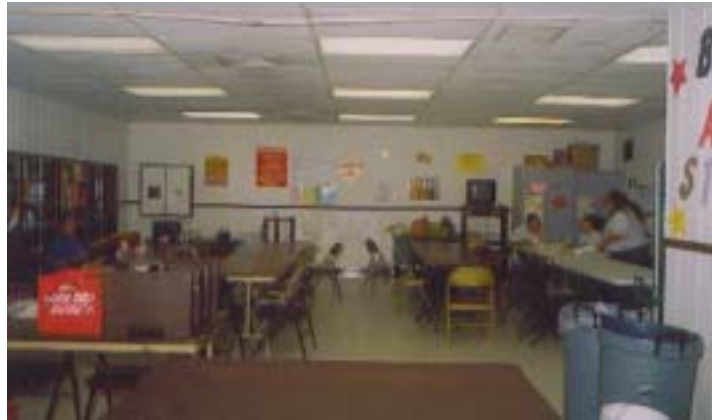
The Marktown Community Center after the most recent repairs. While those responsible for the work did not come nearly close to our expectations, I suppose we should be satisfied with a coat of paint, some new lights and a few new book cases. Maybe if we had all been permitted to work together on the proposed New Marktown Community Center, we wouldn't have to settle for the leftovers and scraps.
