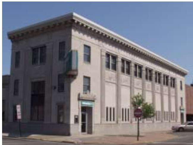
The First National Bank in Indiana Harbor still stands today. The question is, how long will it remain?
