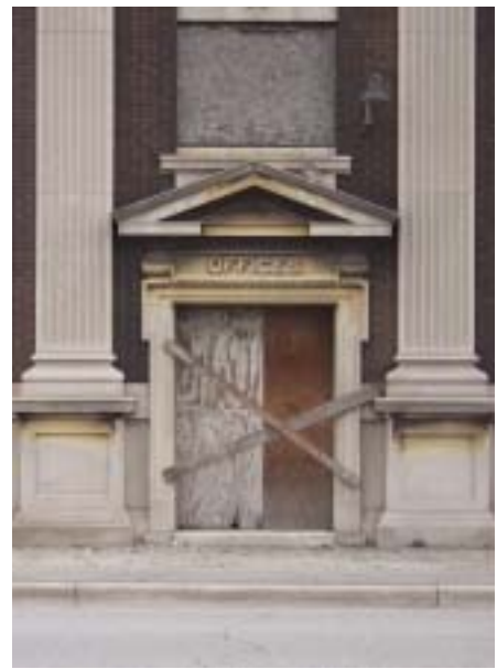
Above: While simpler in design than the main entrance, the office entrance was the only access to the second floor.
