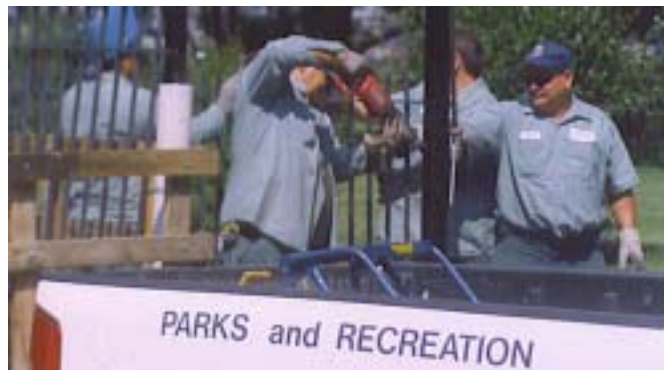
Parks Department workers install the new gate and fence designed to protect our parks.
